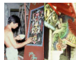
Paintworks on timber - Kun Ting Study Hall (Left), Tai Fu Tai (Right)
