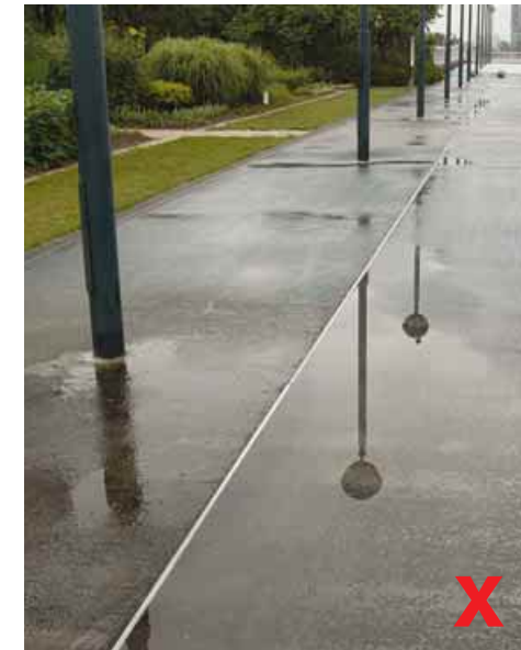
3.1.4.1b Water ponding along tactile cue on walkway is hazardous to users
