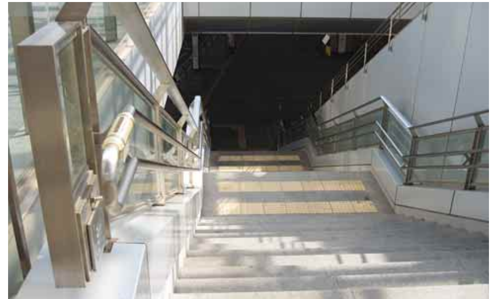
3.1.6.1d Staircase with tactile warning strips, railings on both sides and Braille on the railing horizontal extension
