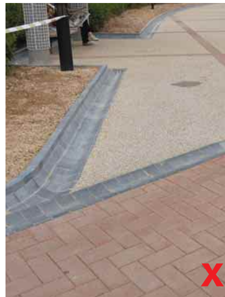
3.1.4.2c Uncovered surface channels on accessible routes are hazardous and should be avoided
