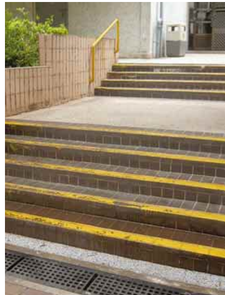
3.1.3.3b Markings should be properly maintained, worn-out markings should be repaired or replaced immediately
