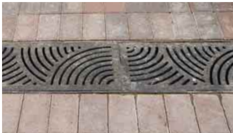
3.1.3.1a Channel cover levelled with floor surface and gaps at the gratings are less than 13mm wide
