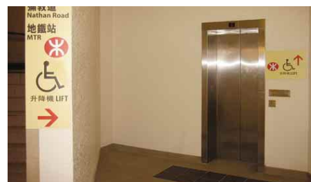
3.1.6.1g Signage and tactile strips leading to an accessible lift
