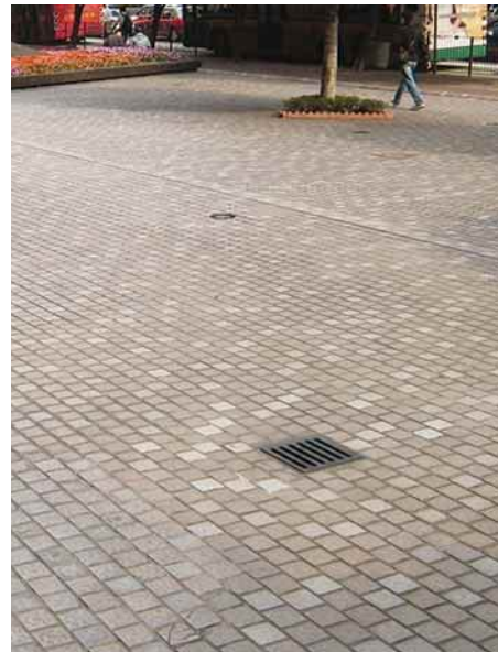
3.1.4.3b Floor drains covers flush with adjacent floor surfaces with slots less than 13mm wide
