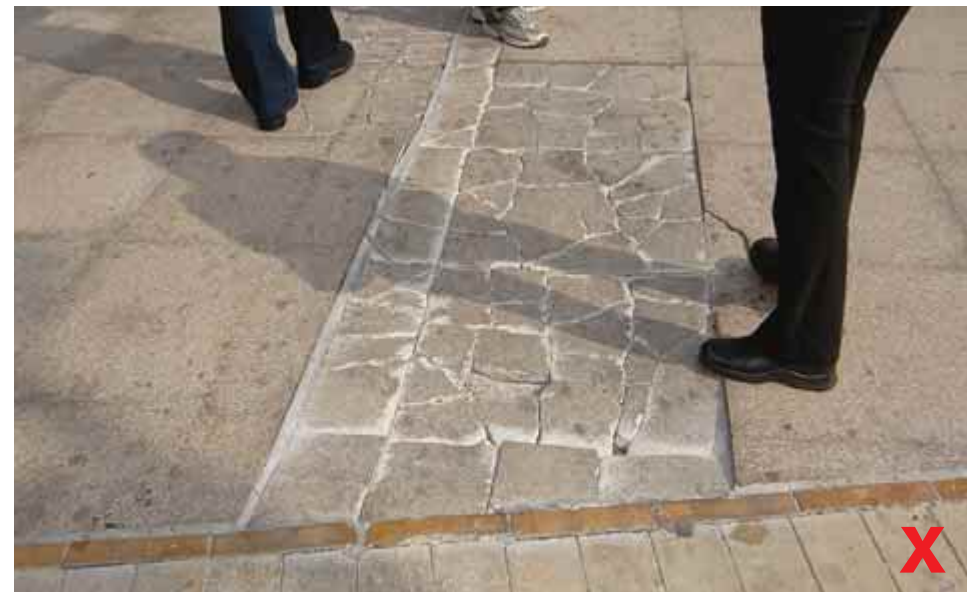
3.10.2a Damaged areas should be properly fenced off and the travel path properly re-diverted
