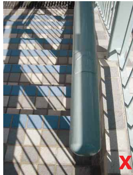
3.2.3.1e Busy floor patterns combined with lighting effect can cause discomfort and hazard to users travelling on the staircase
