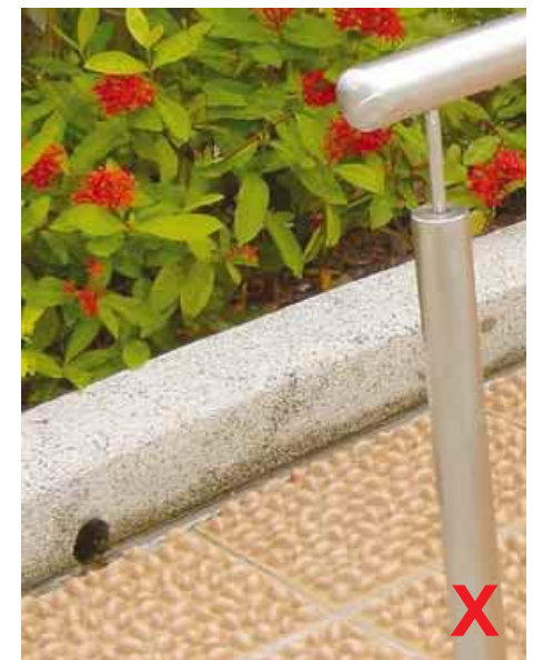
3.4.3.2c Weep-hole outlets should not be positioned directly at ground surface of outdoor exercise areas
