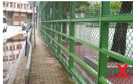
3.4.1.1 d Properly supported chain-link fence (top) and deformed chain-link fence protruding onto a narrow footpath (bottom)
