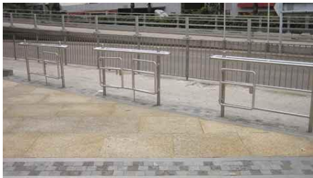
3.4.1.3a Wide opening in between guardrails
