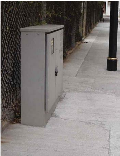
3.4.5.1b Utility control box placed on the edge of the walkway
