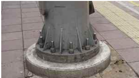
3.4.1.4c Lamp pole with wedges set on plinth to avoid tripping
