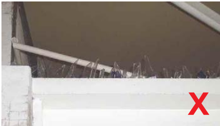
3.4.1.1b Avoid the use of broken glass as anti-climbing device
