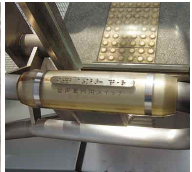
3.6.4.3b Handrail fitted with sensor giving both tactile (Braille) and audible (taped message) information when the hand is placed on it
