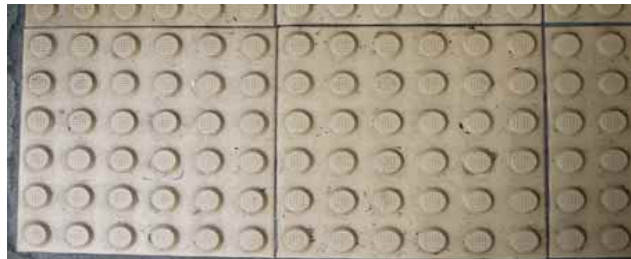
3.6.2.1b Hazard warning tile with raised dots arranged in square grid parallel to the sides of the tile, laid perpendicular to travel direction
