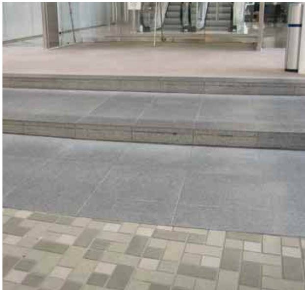
3.9.3.1a Change in flooring materials with gradual change in slip resistance at entrance area from external ground
