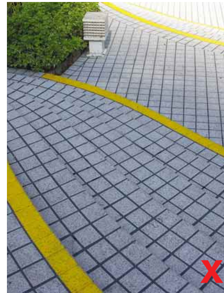
3.9.2.1g Steps without buffer zone and conspicuous nosing are hazardous
