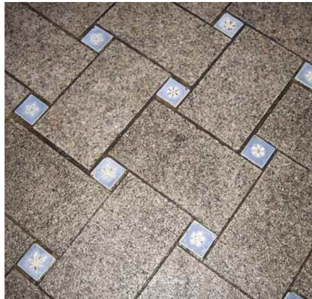
3.9.3.1b Slip resistance of small inserts is equally important
