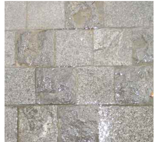
3.9.3.1c Strike a balance between good slip resistance and tripping hazard when considering the surface roughness of a flooring material
