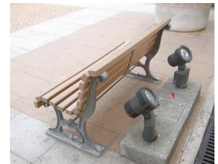
4.4i Lighting fixtures mounted on a plinth hidden behind a seating bench
