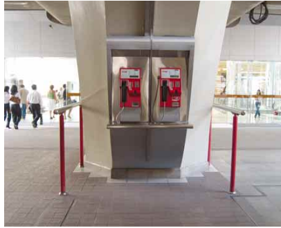
4.4u Telephones mounted underneath a staircase with protective rails provided on both sides
