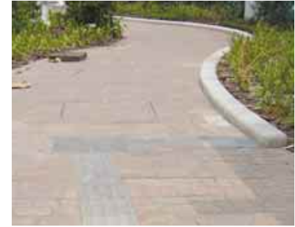
4.6m Detectable surface switching from a tactile guide path to a kerb; users should be adequately alerted to such change in detectable cue
