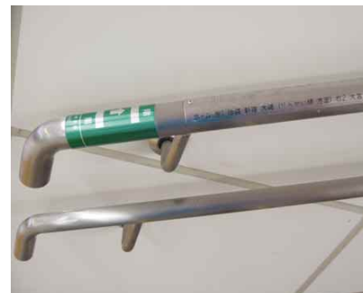
4.6s Braille information on top handrail to identify the location and indicate travel direction
