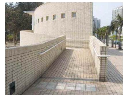
4.7mm Visual contrast created by using different finishing materials between the floor and wall of ramps
