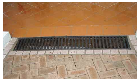
A2.3.6b Channel covers with slots greater than 13mm may trap wheelchairs or walking canes
