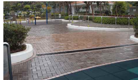
A2.3.6a Surface channel flush with adjacent floor surfaces for collection of rainwater
