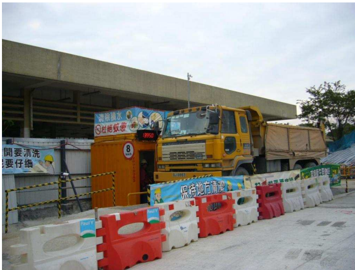
Photo 15. Provision of Weight Bridge with CCTV system
