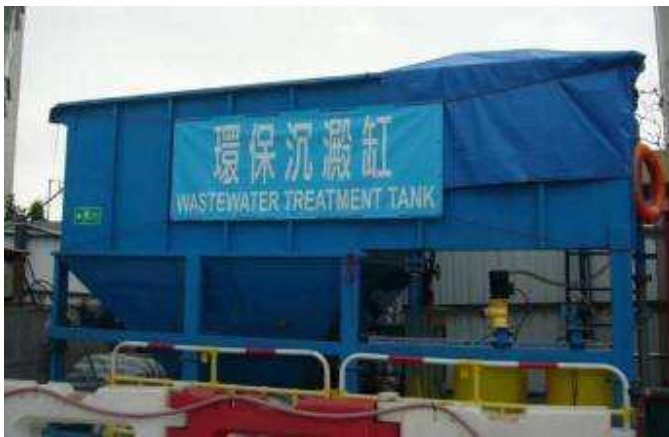
Photo 8. Wastewater treatment system (Aqua-Sed) was provided on site
