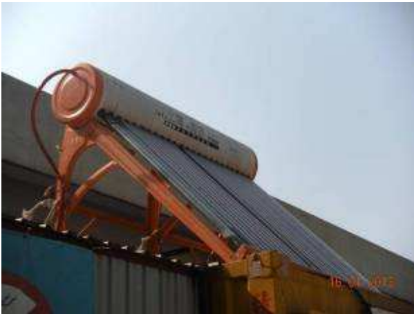
Photo 20. Solar energy heating system
