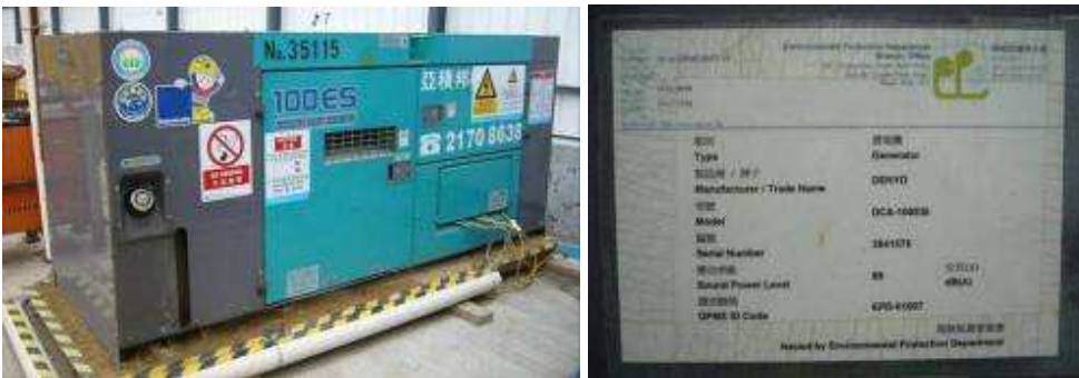
Photo 11. Provision of Quality Powered Mechanical Equipment (QPME)
