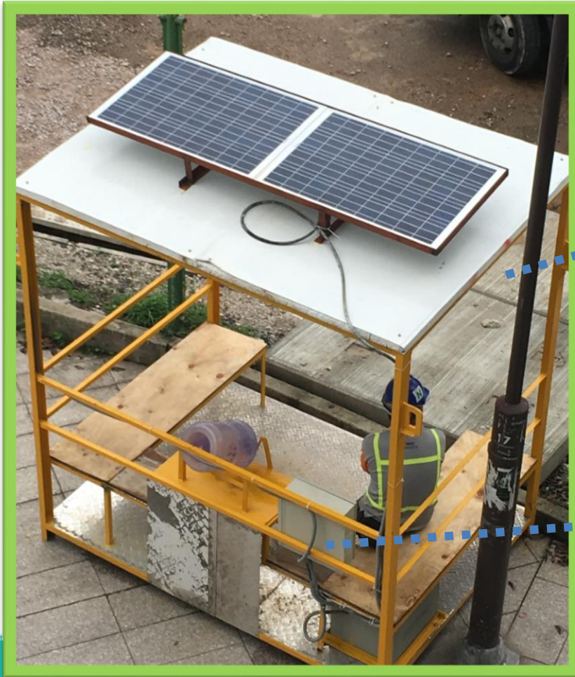
Solar energy for moveable workers rest area
