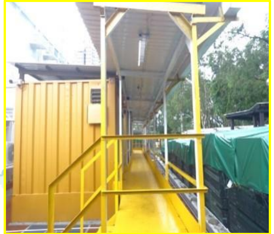
Motion sensors for lighting system
