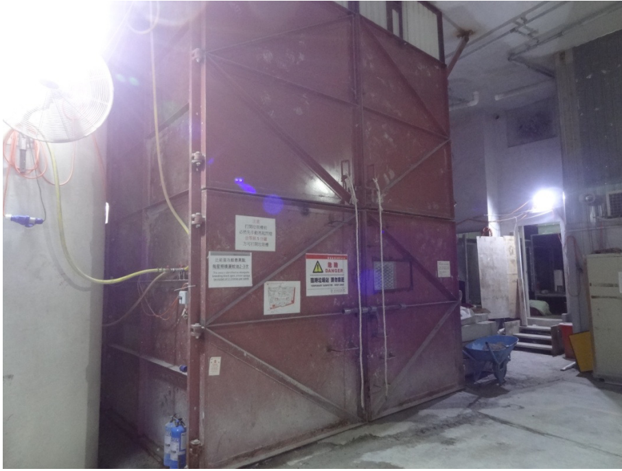
Totally enclosed refuse chute with built-in automatic water spraying system
