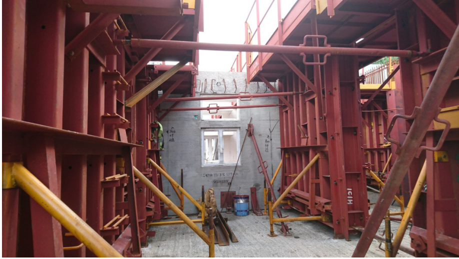
Extensive use of metal formwork in typical floor to replace use of timber
