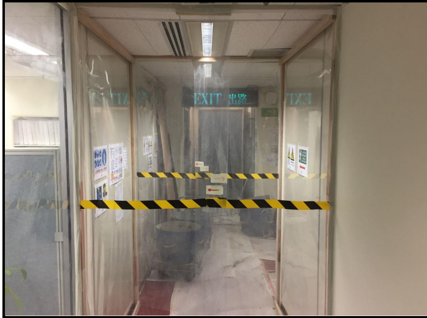
Dust Lobby (Dust Screen) to provide safeguard against outspread of dust.
