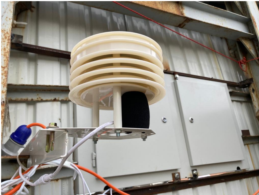
Sensor installed near by ASR/NSR
