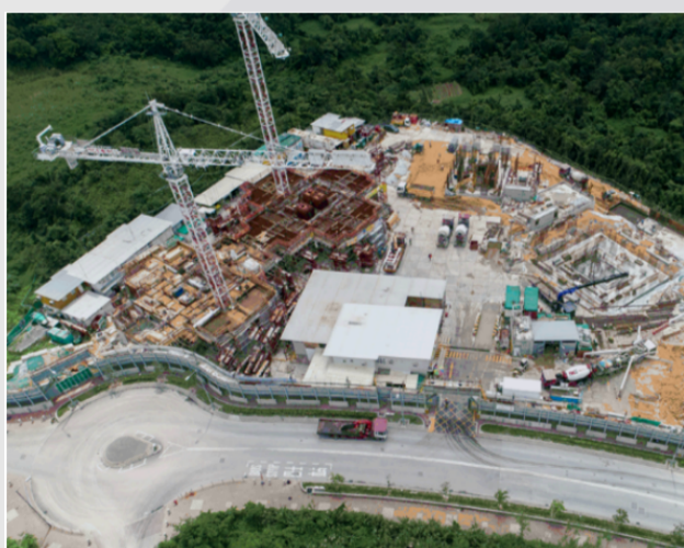
The construction site of the Disciplined Services Quarters for the Fire Services Department at Pak Shing Kok in Tseung Kwan O
