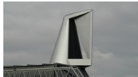
▲ Application of Windcatcher
