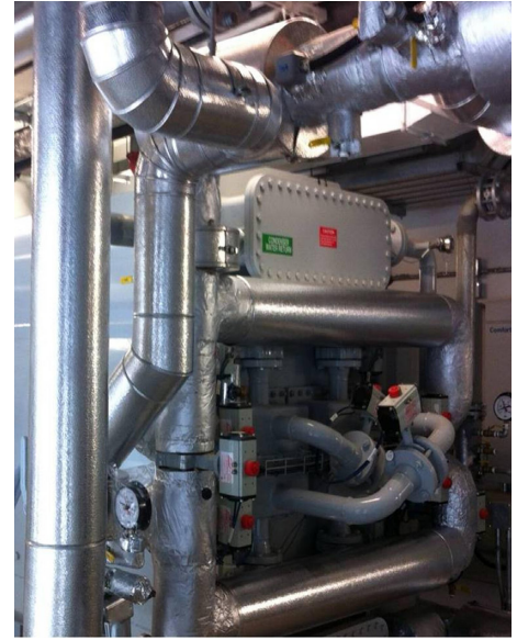
▲ Bio-diesel Generator and Absorption Chiller
